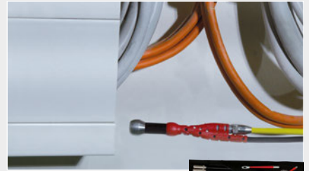
Shafts and underfloor ducting
